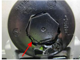
Cracked Filter Cap
